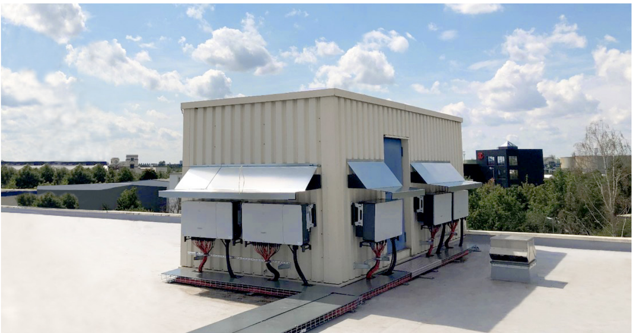
Fig.6 AC 500kW Rooftop PV Plant in Germany
